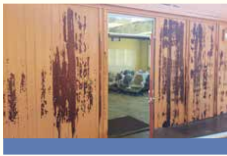
Some College of Marin facilities are in need of repairs to provide safe, well-maintained learning environments.
