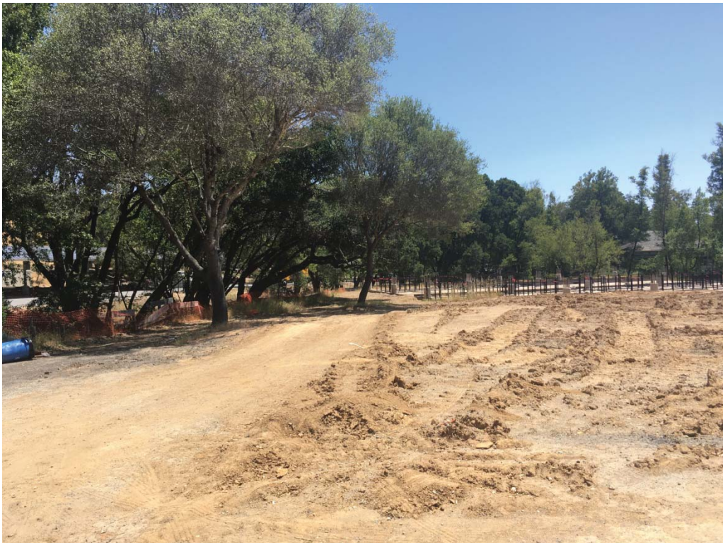
Photo 4. Northern edge of Jonas construction site, view of site of future creek crossing for raised footpath (6/7/2018)
