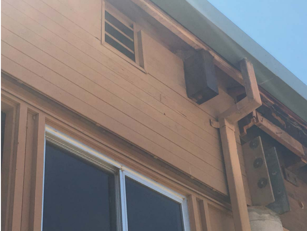
Photo 7. Swallow nest under eaves of Jonas remaining building (6/7/2018)
